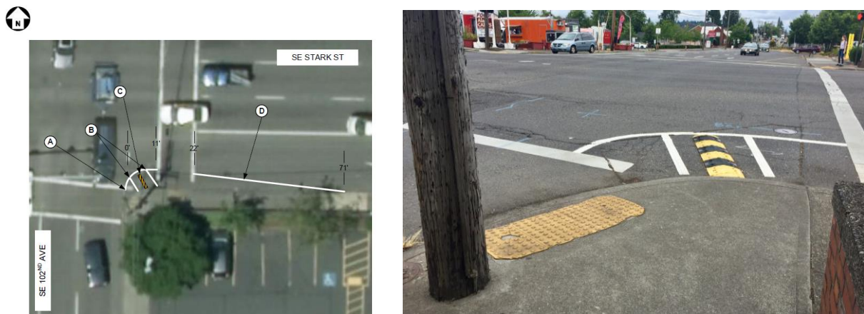
Figure 9. A PBOT work order (left) shows a top-down view of a wedge with thermoplastic striping on the southeast corner of SE 102 nd Ave. & Stark St. The photo (right) shows the installation looking north/northwest.
