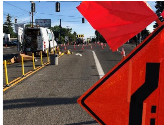
Figure 14. High-volume intersections such as SE 122nd Avenue & Market Street can require significant traffic control.
